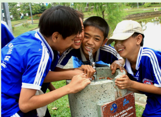
"Safe Water Declaration" was presented on the occasion of the centenary of HueWACO foundation
