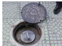
Manhole for direct sewage portable toilet
